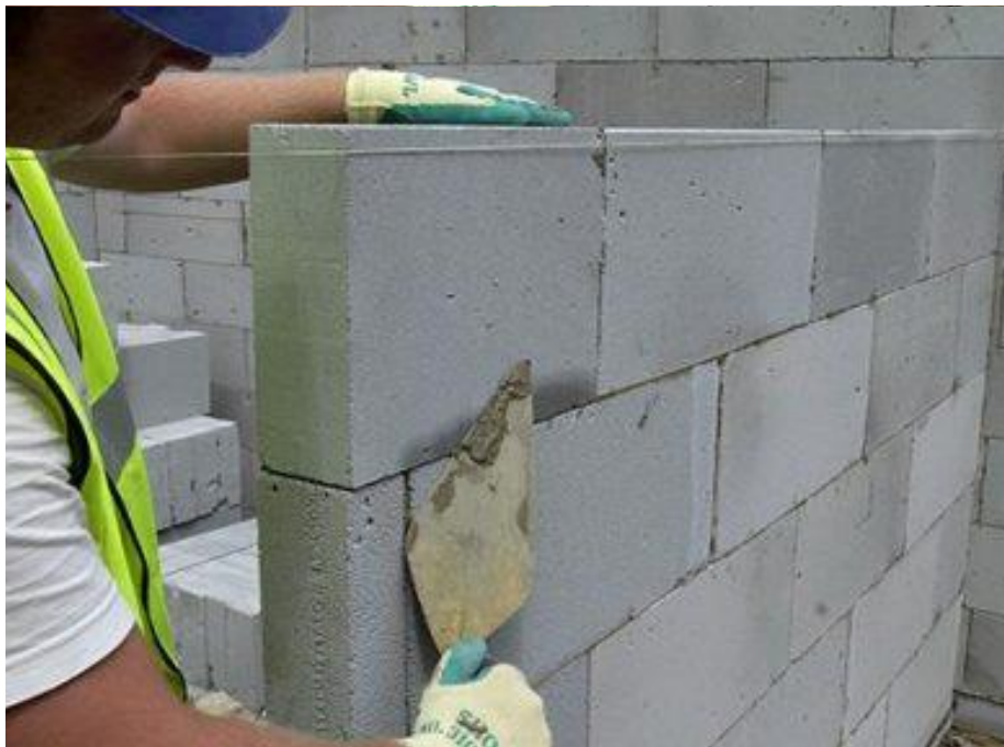
200 mm Autoclaved Aerated Concrete (AAC) with 15 mm plaster on both side U Value 0.77 \text{ W/m}^2\text{K}
