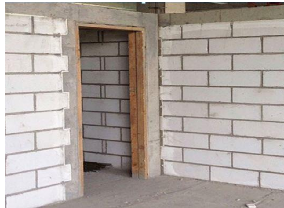
300 mm Autoclaved Aerated Concrete (AAC) with 15 mm plaster on both sides U Value 0.54 \text{ W/m}^2\text{K}
