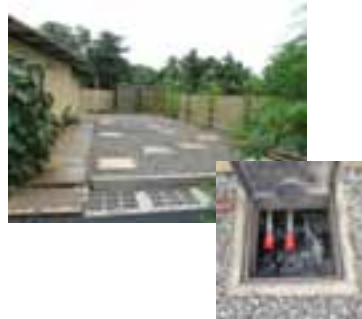
Waste water treatment system
