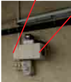
Figure 2.3a Temperature humidity logger assembly for monitoring ambient conditions
