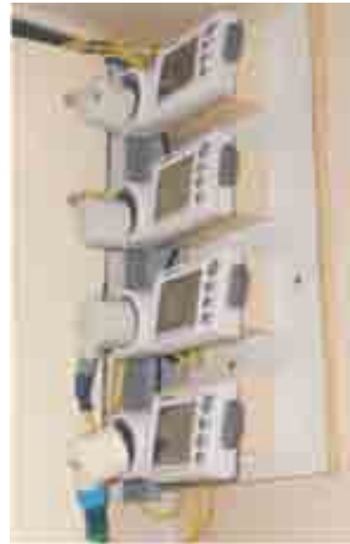
Figure 2.3c Energy loggers for monitoring electricity consumption of air-conditioners and geysers
