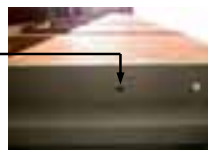
Ventilation sleeve for the cavity
