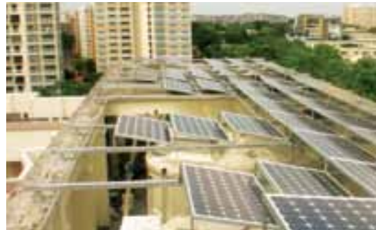
Figure 8.5 Solar PV system on a rooftop
